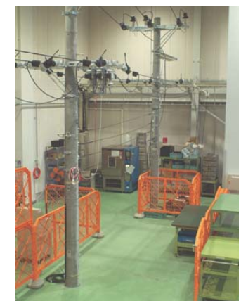
Simulated power pole for electricity distribution line
